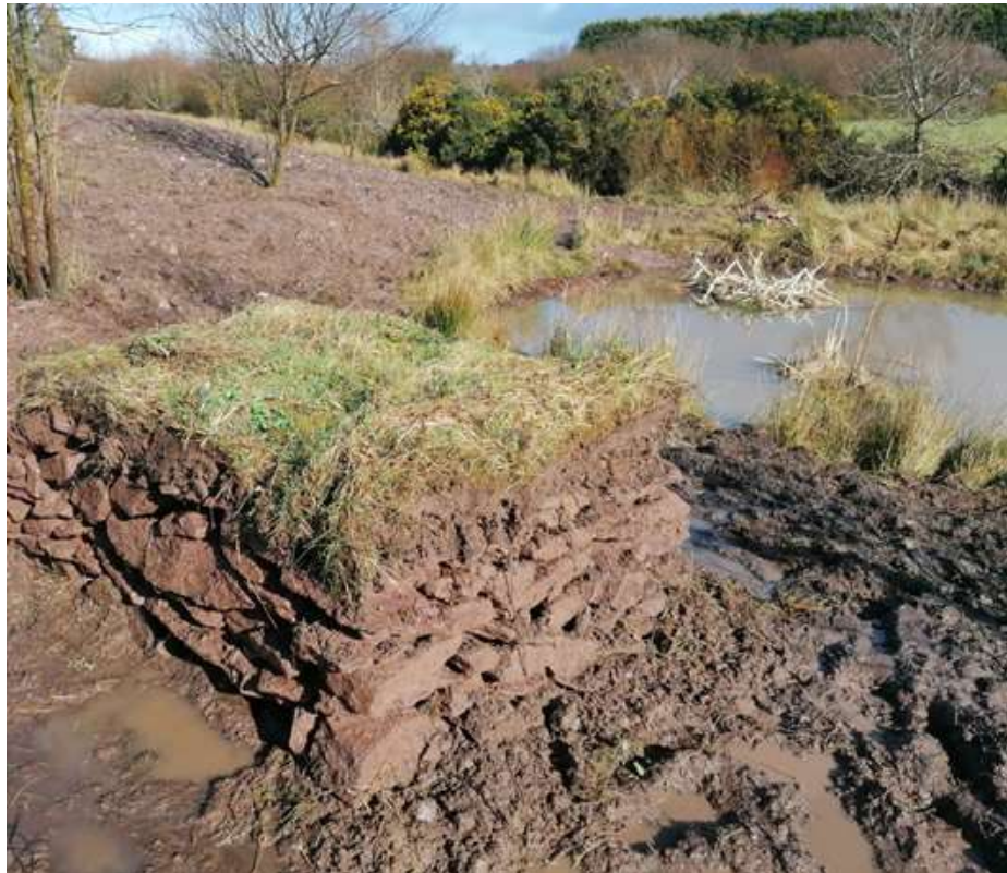
Hibernaculum construction adjacent to a Smooth Newt pond (Source: Trituris Environmental Ltd.)
