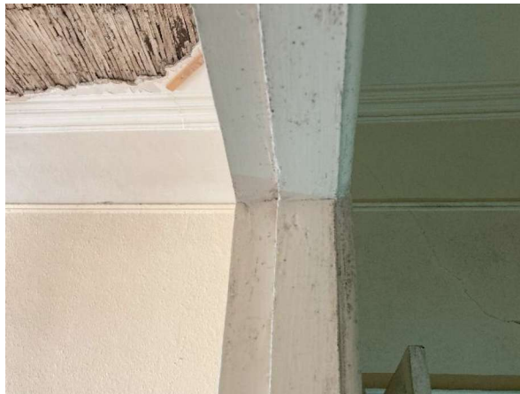
Modern partition breaking through cornice.
