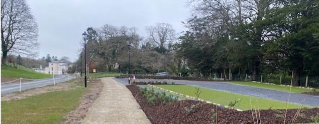
Car parking bays with grass-grid finish at the new avenue car park
