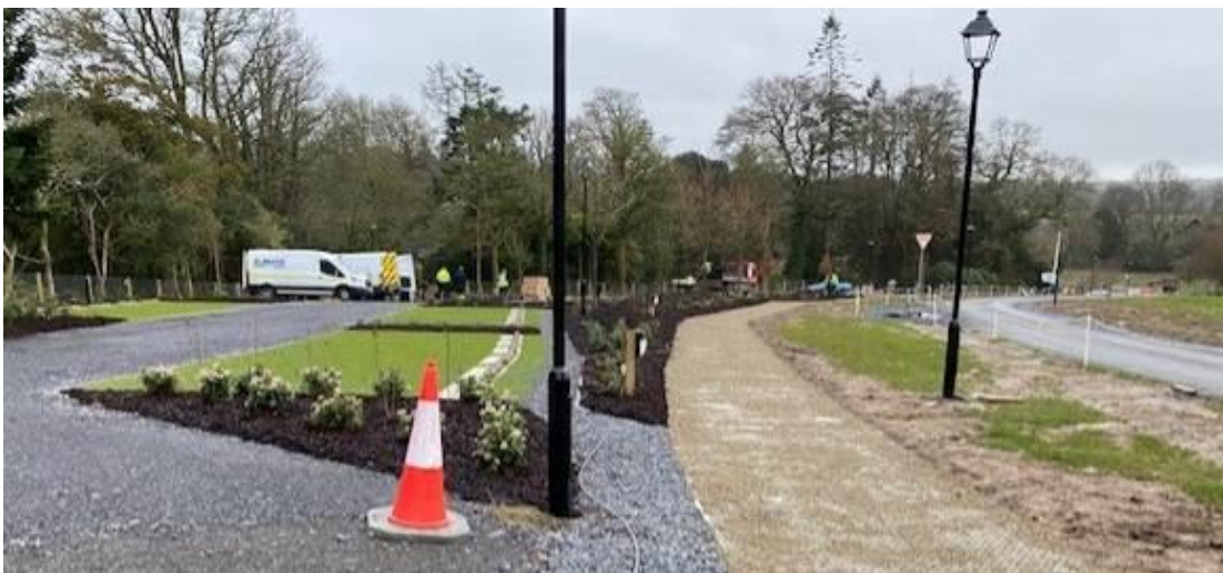
Car parking bays with grass-grid finish at the new avenue car park
