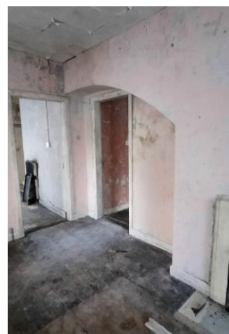
The building is not currently habitable
