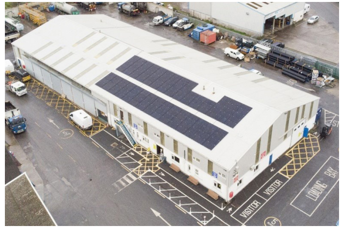
Figure 3. Solar Array on Dungarvan Depot
